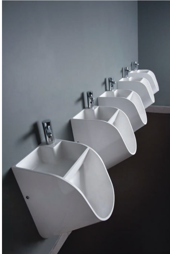
Fig. 16.11 Urinals with sink for flushing
