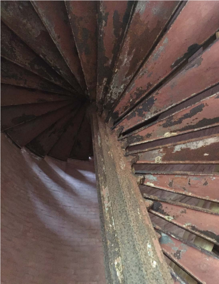
Open-tread iron stairs of the 1857 light spiral to the masonry watch room and iron lantern above.
