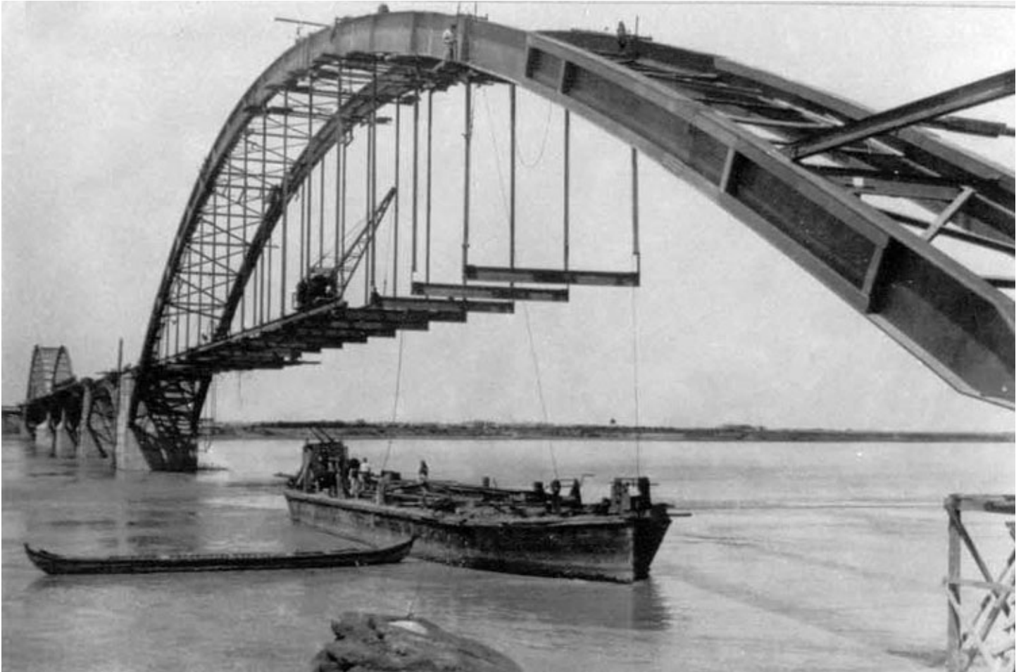
A 1930s picture of the White Bridge using barges in the constructing process.
