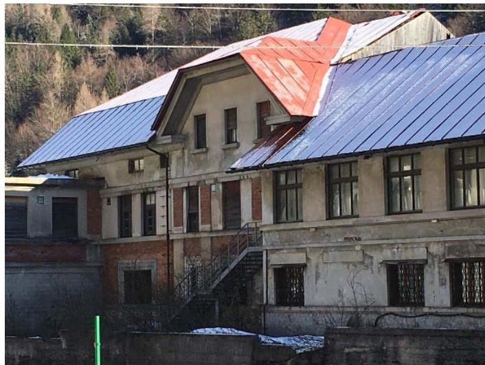
The workers’ recreational club, late 1920s, designed by architect Cesare Miani, is in a state of dereliction, as are most of the surrounding buildings.
