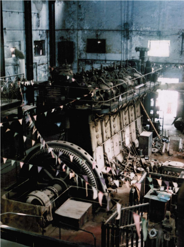
Diesel Power House with Ship Engines manufactured in Winterthur, Switzerland
