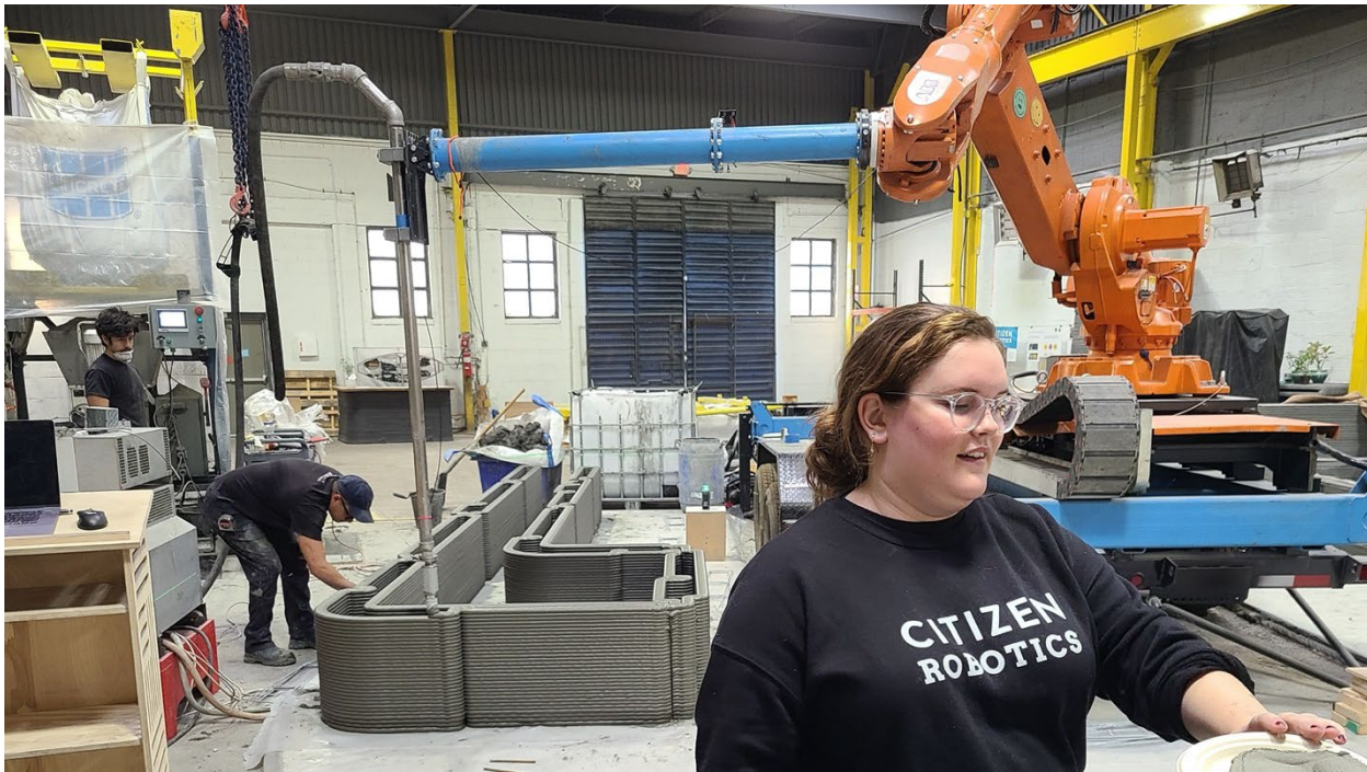
Figure 6: The components for the Sheridan Residence - the first project realized by Citizen Robotics and the first 3d printed home in Detroit – will be fabricated off-site and then shipped for installation. Over time, this method could greatly decrease the costs associated with home construction. (Image courtesy of Citizen Robotics)
