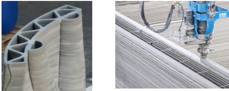
Figure 1: A concrete bead ties together the exterior and interior 3d printed walls (left, image source: Suntharalingam 2021) and standard steel reinforcement to tie together the exterior and interior 3d printed walls (right) Source: PERI
