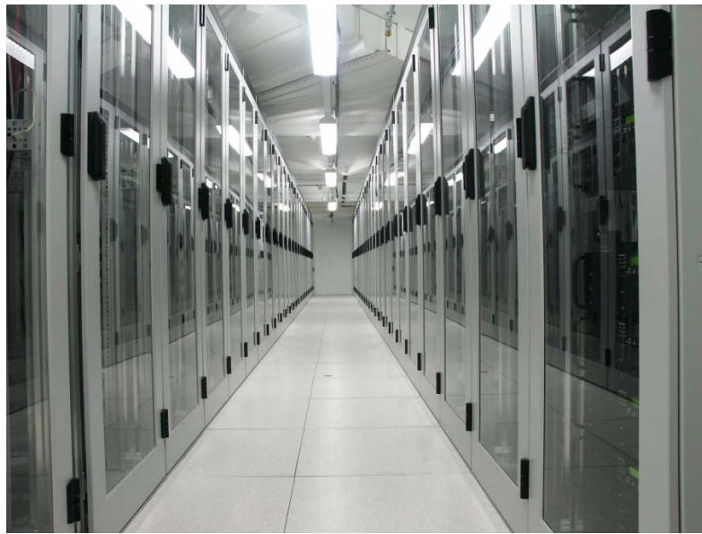
Figure 2 Taken from http://press.1and1.com/uploads/press/images/Server_room_1.jpg
