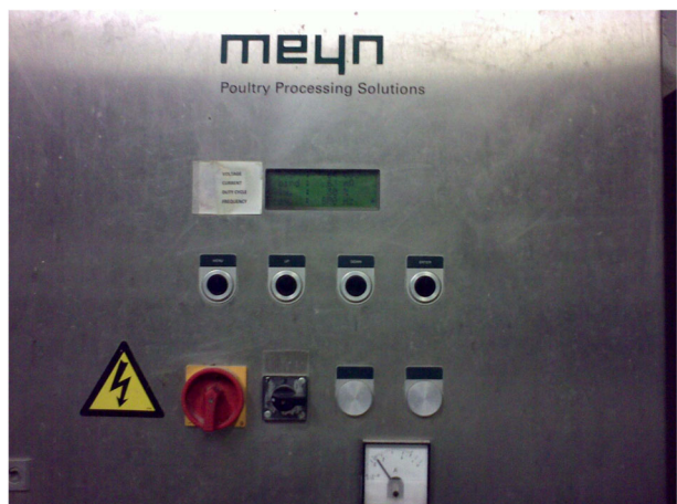
Fig. 5 The electric panel that control the method of stunning
