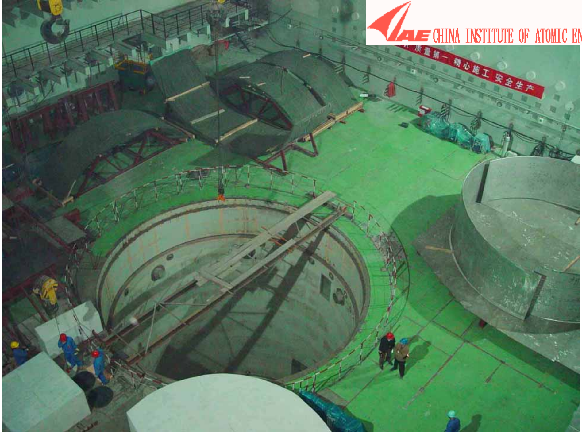
Reactor Pit and Some Parts of CEFR Main Vessel (2005.04)
