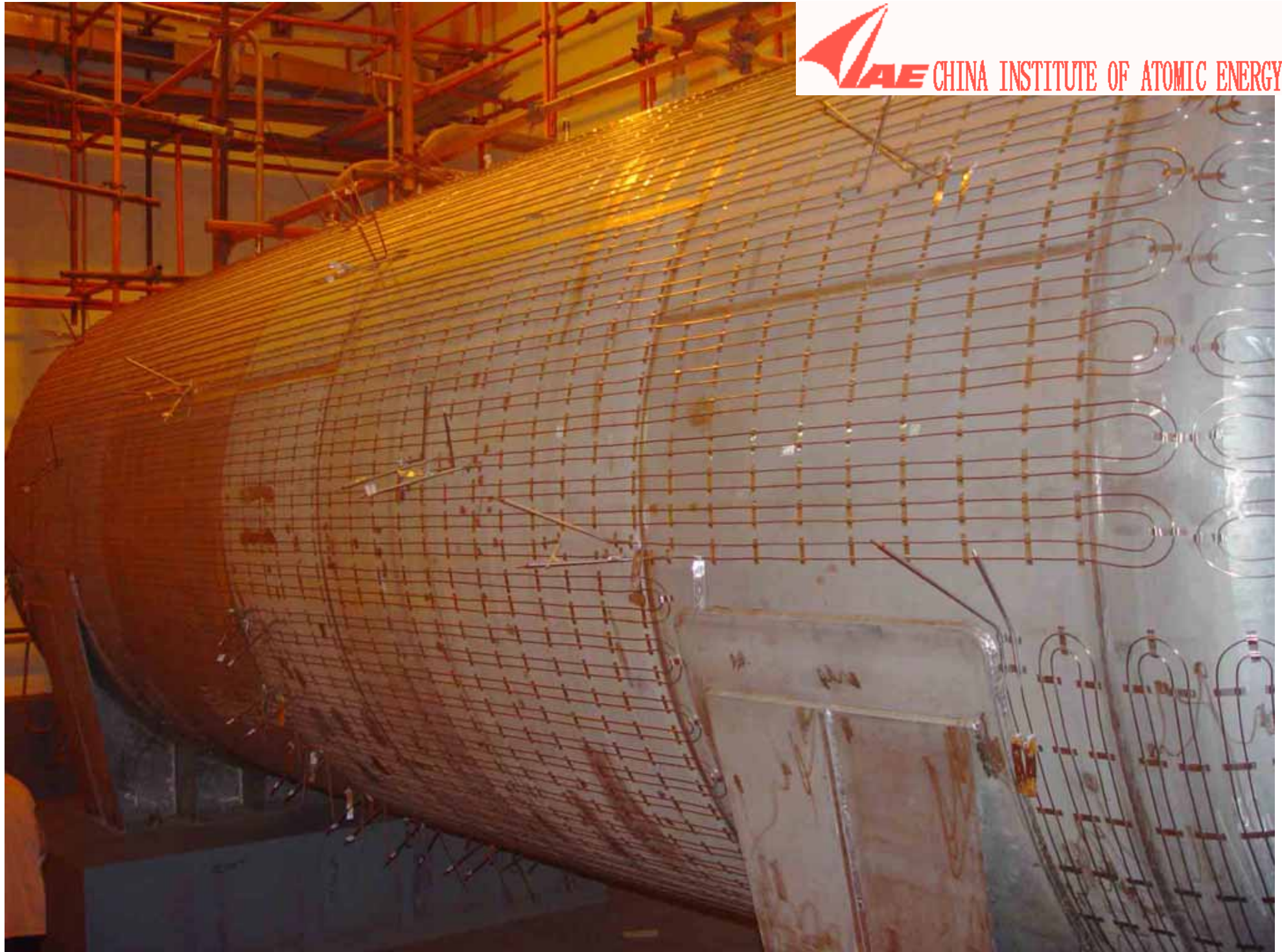
One of Five Sodium Storage Tank (2005.02)
