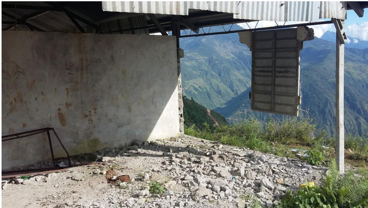
Figure 5.4. In Listi, a building lost most walls in the earthquake while a window-shutter holds on (Photo credit: author, 2017).
