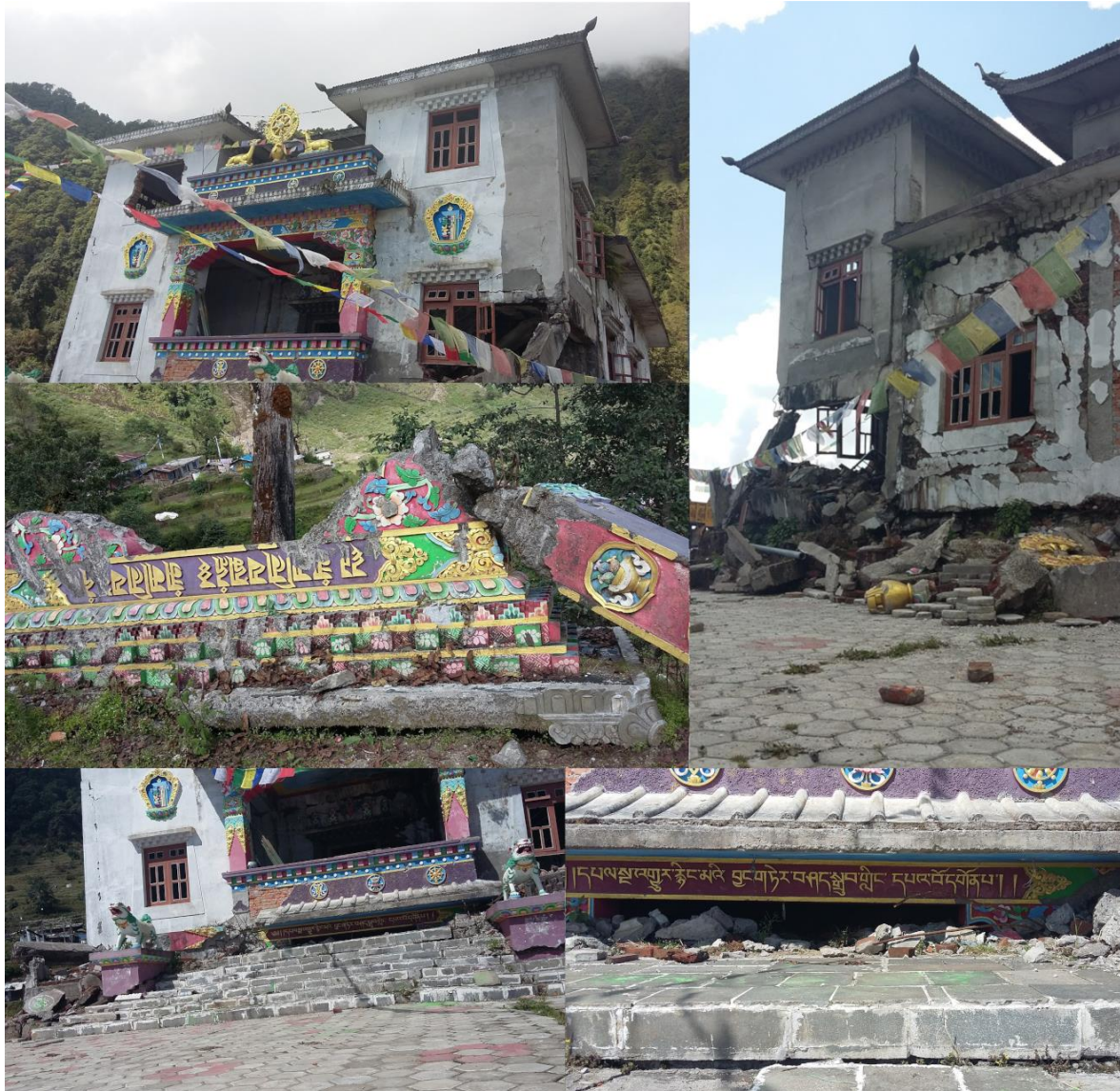
Figure 5.8. A collage of images from Listi-Gumba where the village's Gumba (Temple) was destroyed by the Gorkha earthquakes (Photo credit: author, 2017).
