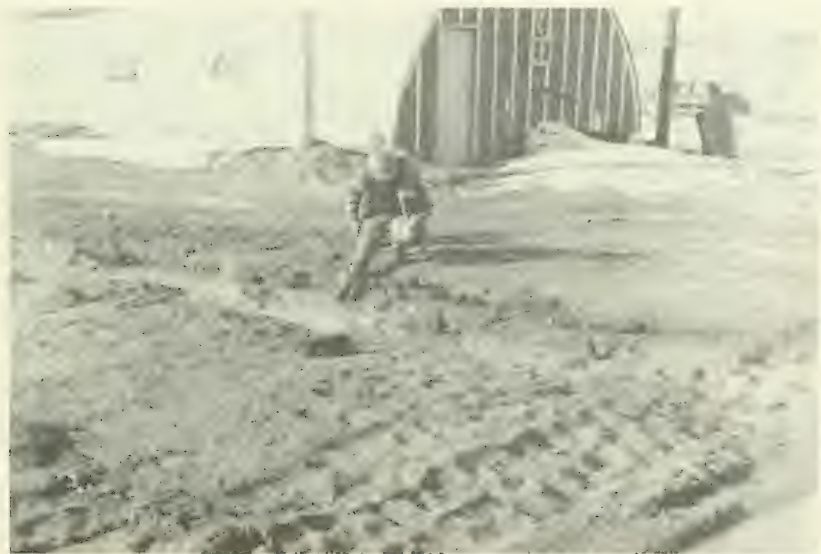
2. Slump in gravel on street in Barrow, where steam line produced thawing of permafrost. Photographed May 12, 1950.
