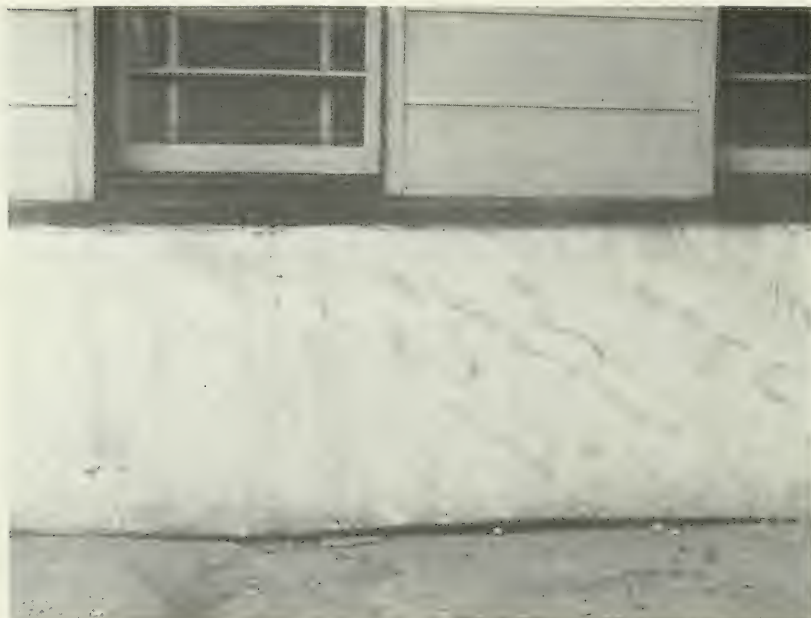
2. Settling cracks in foundation wall of the U. S. Post Office, Nome, Alaska, after thawing of permafrost under the building. Photographed August 10, 1948.
