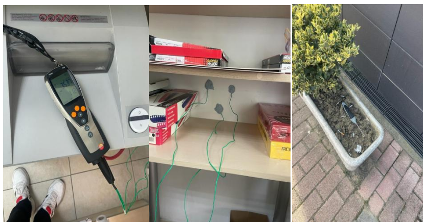
Figure 4. A. Testo 435-2 measurement device during first measurements. B. Internal sensors C. External wireless sensor; source: authors
